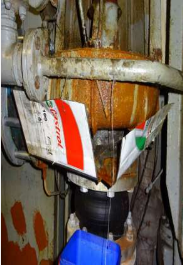
Corrosion due to leaking machinery pump and illegal drip pan/bucket underneath
