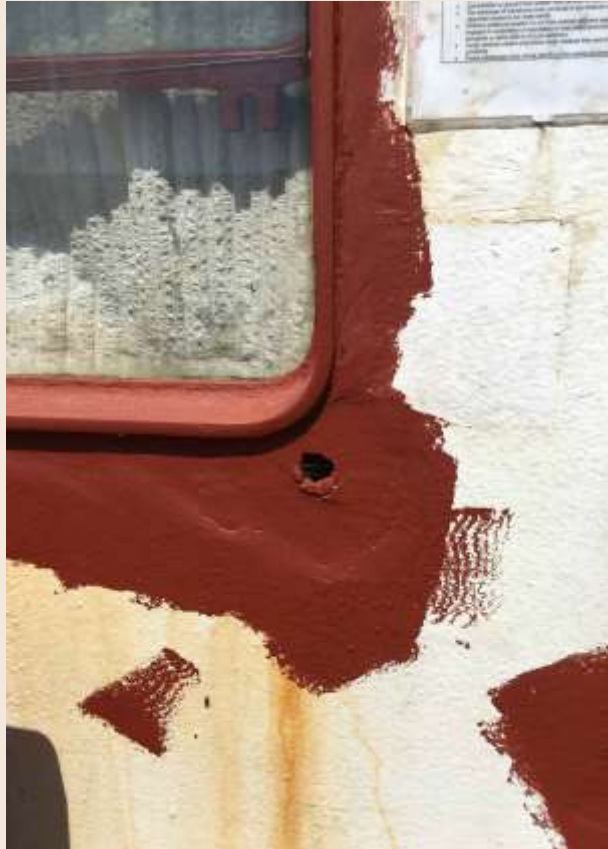
Hole on the accommodation structure
