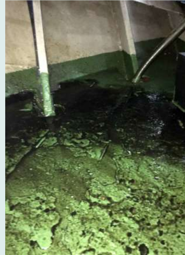
Oil on engine room flooring
