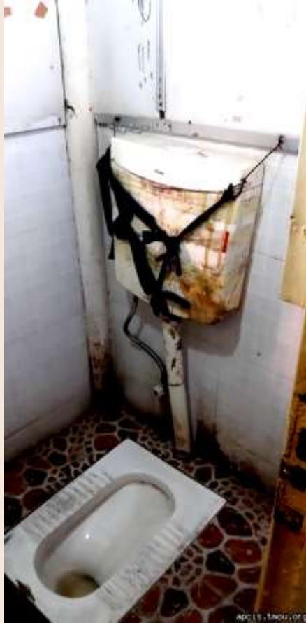
Damaged toilet flush tank
